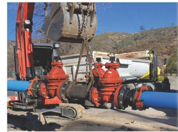
Project Managed by LSDA Administration; Quail Trail Water Line Replacement: Installation of 3-valve assembly at the intersection of Spring Valley Road and Quail Trail.
