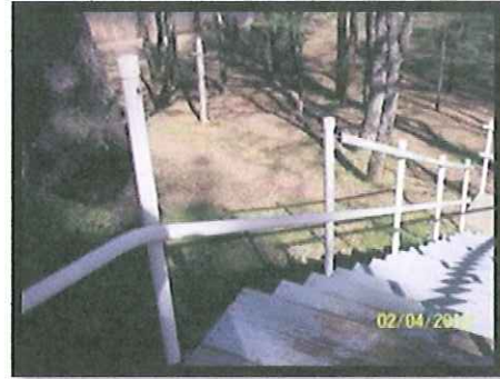
Missing Section of Upper Railing
