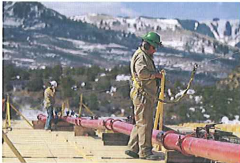
A worker helps monitor water pumping pressure and temperature, at the site of a natural gas hydraulic fracturing and extraction operation run by Encana Oil & Gas (USA) Inc., outside Rifle, in western Colorado. A doubling of water prices wouldn't hurt energy operations, but soaring prices would.
