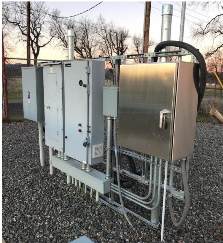
Figure 1 - New Power Panel
