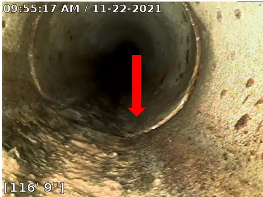
Figure 1: Camera-inspections on Deer Hill Rd customer lateral reveal leaking joints and heavy water intrusion.
