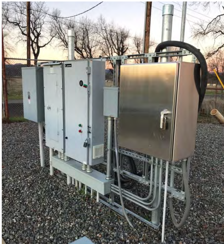
Figure 1 - New Power Panel
