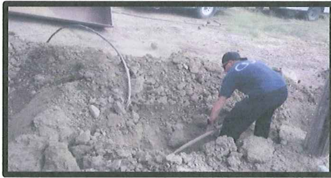
Deerhollow - push through for a service connection. Old service connection was leaking.
