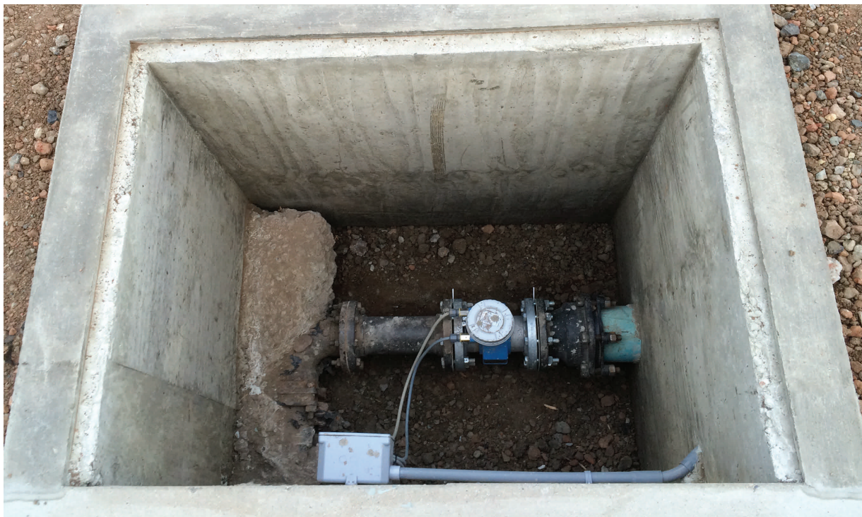
New flow meter to WWTP Inflow
