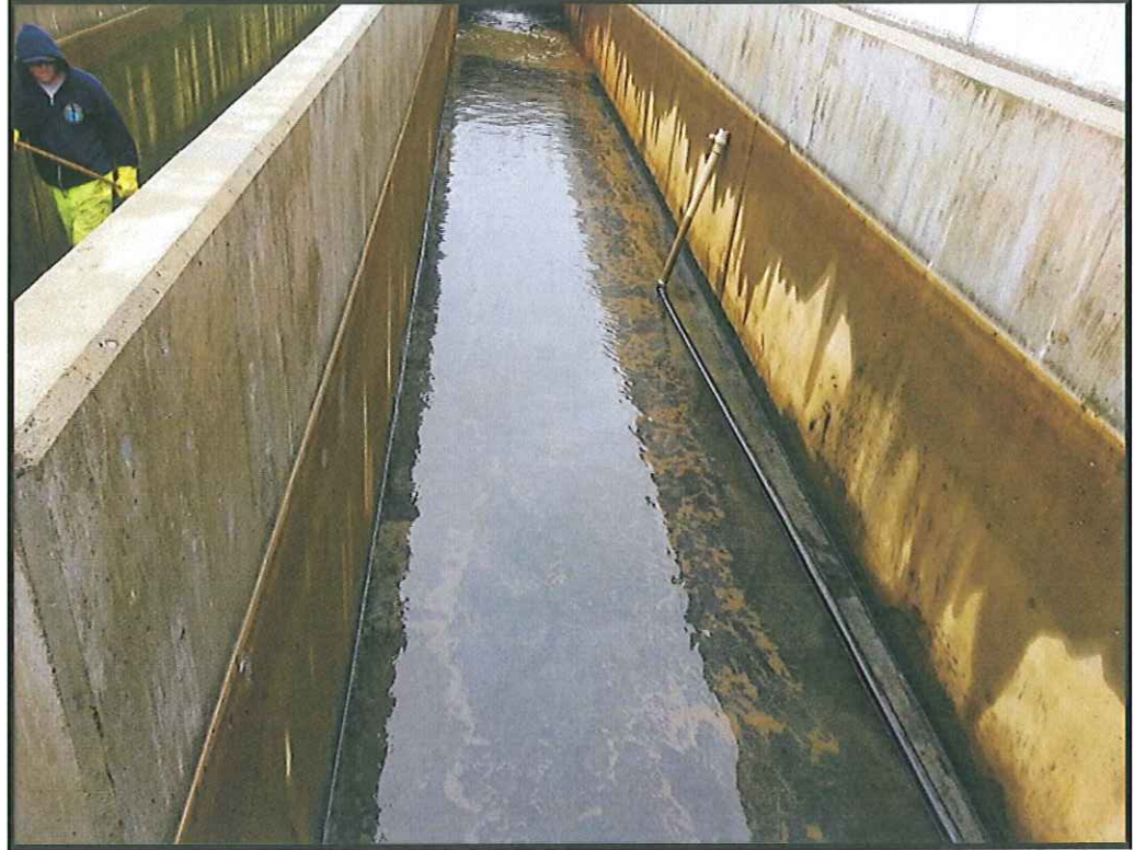
Chlorine Contact Basin after routine cleaning.
