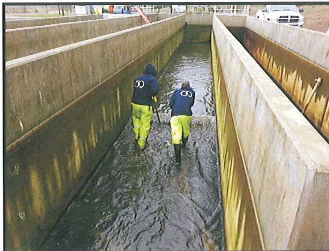
Field Operations staff cleaning Chlorine Contact
