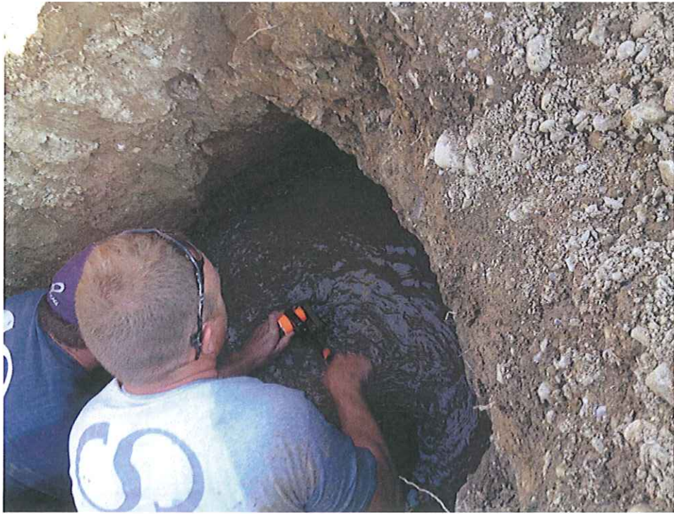
Emergency repair work being performed on District's mainline off of Moonridge Road.
